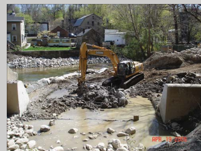
Breach of spillway almost complete.
