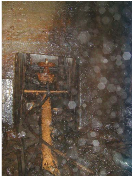
Photograph No. 21 Rusted gate valve located at bottom of concrete plug in the abandoned low-level outlet tunnel at Copco 1 Dam. Bureau of Reclamation - Pacific Northwest Underwater Inspection Team. Copco 1 Dam, Klamath Hydroelectric Project, Oregon-California – April 12-16, 2010.
