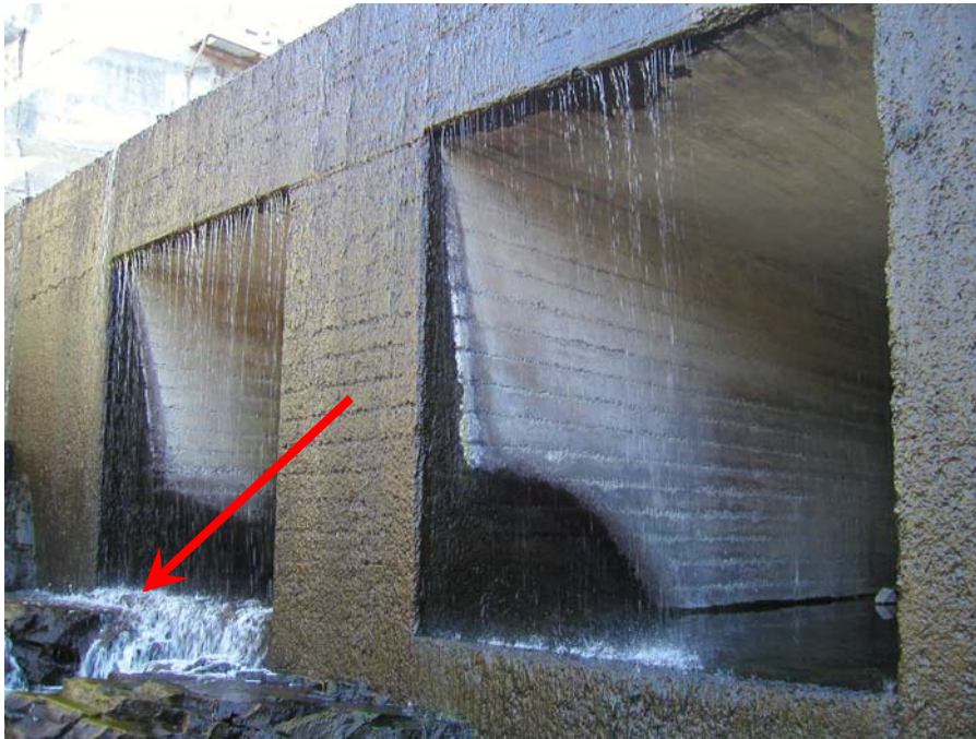
Photograph No. 28 Close-up view of double barrel diversion conduit exit. Note surface flow exiting right side conduit (red arrow). Stop logs on right side are racked in the guide slot causing leakage. Significant P-Delta effects were noted by divers at this location. Extreme caution and distance should be maintained by any future dive team to this area. Bureau of Reclamation - Pacific Northwest Underwater Inspection Team. JC Boyle Dam, Klamath Hydroelectric Project, Oregon-California – April 12-16, 2010.
