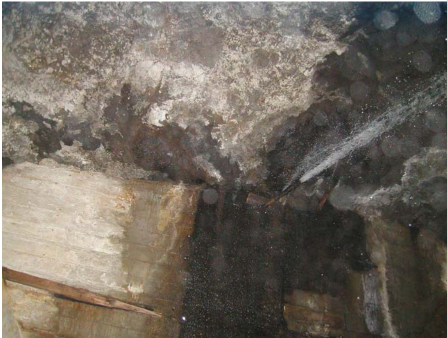
Photograph No. 22 View at top of concrete plug. Pipe at top of plug releasing water at approximately 10 to 15 gals/min. Bureau of Reclamation - Pacific Northwest Underwater Inspection Team. JC Boyle, Copco 1 and Iron Gate Dam, Klamath Hydroelectric Project, Oregon-California – April 12-16, 2010.
