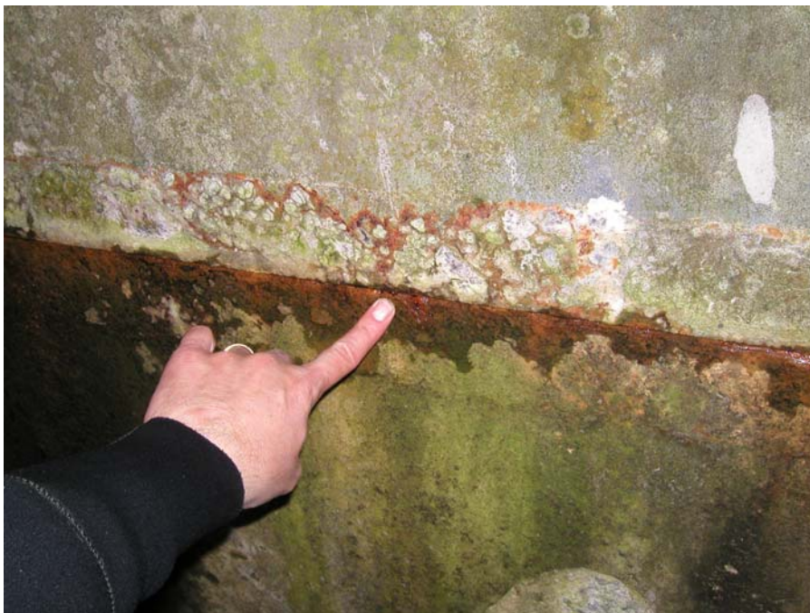
Photograph No. 27 Finger pointing to seepage through horizontal lift line of the stop logs in the left side of the double barrel diversion conduit. Bureau of Reclamation - Pacific Northwest Underwater Inspection Team. JC Boyle Dam, Klamath Hydroelectric Project, Oregon-California – April 12-16, 2010.
