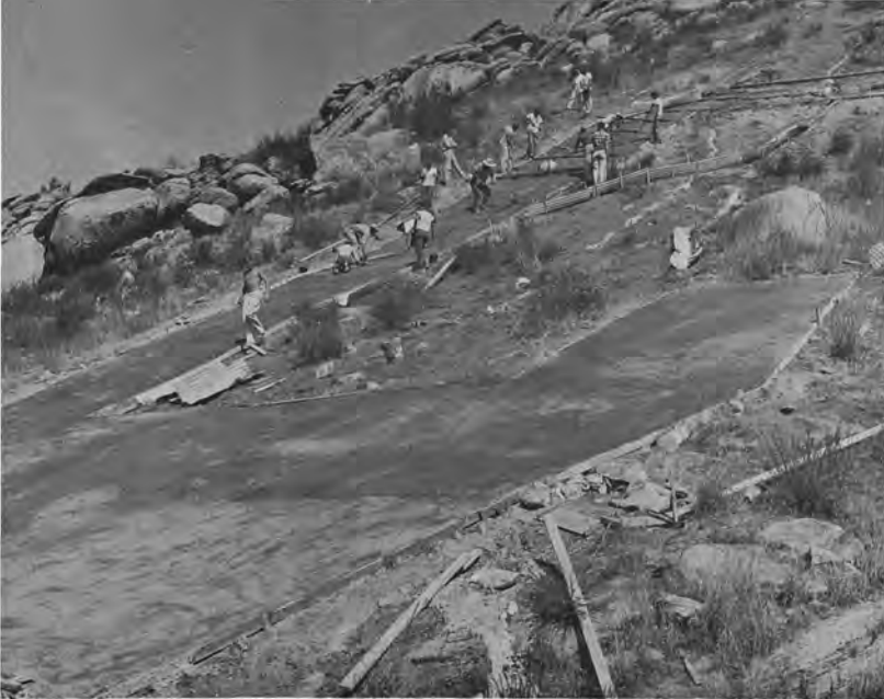
Construction of the Big C took place in 1956 by E. L. Yeager Co. and some football players back for pre-season practice. The corrugated metal troughs carried concrete 300 feet from the ready-mix trucks to the forms of the C.
