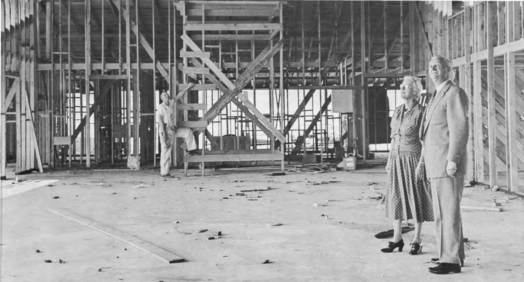
Chancellor Emeritus and Mrs. Watkins surveying the construction of Watkins House, the non-denominational University Religious Center completed in June, 1956 and supported by the community.
