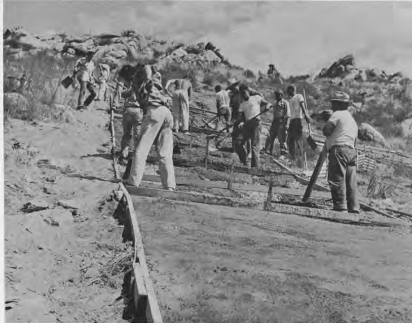
Students and Yeager employees spread concrete into forms as it came rushing down the mountain from the ready-mix truck (skyline-center right). Temporary restrainers were used to slow the flow of concrete.
