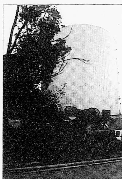
TETSUYA KOSAKA/New University UCI uses a thermal energy storage tank to conserve electricity.
