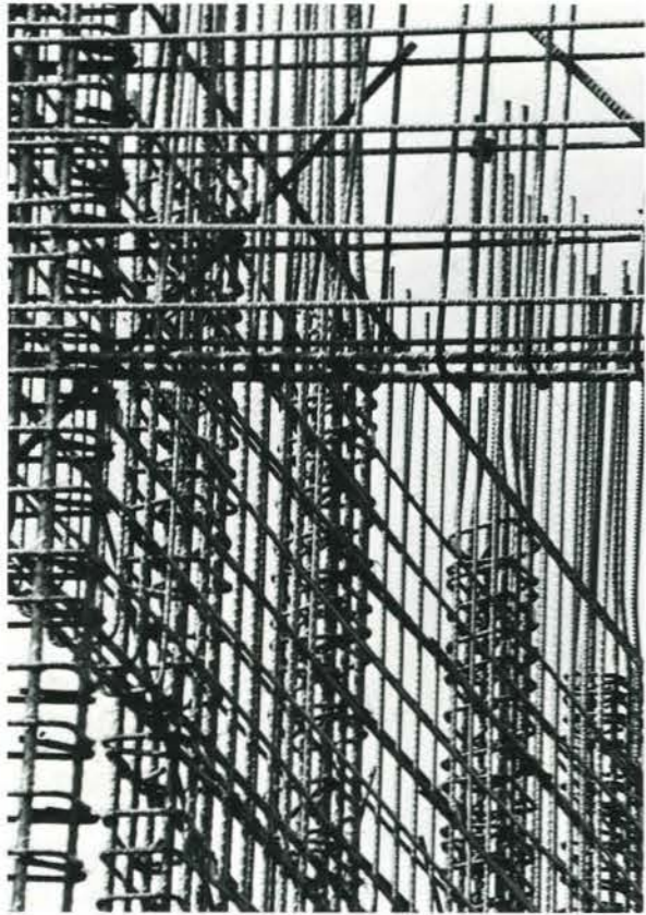
Steel girders reach to the sky and take on an artistic form, almost with a peculiar sort of beauty.
