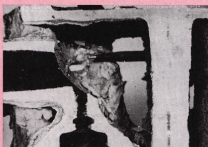
Fig. 12 Lime deposits in the cylinder head from hard water.
