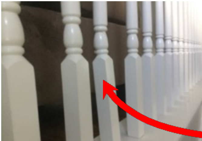
Hallway/Stairway Railings Cracked
