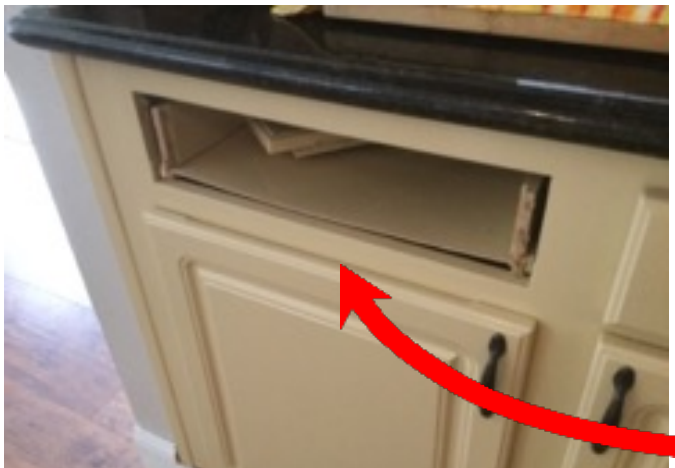
Kitchen Lower Cabinets Missing cabinet door
