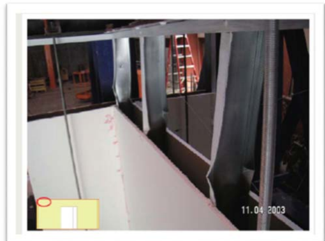
Figure 8. Buckling of studs for a fixed connection partition wall.
