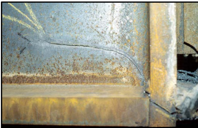
Figure 11. Test data for a pre-Northridge brittle connection (Engelhardt and Sabelli, 2007)
