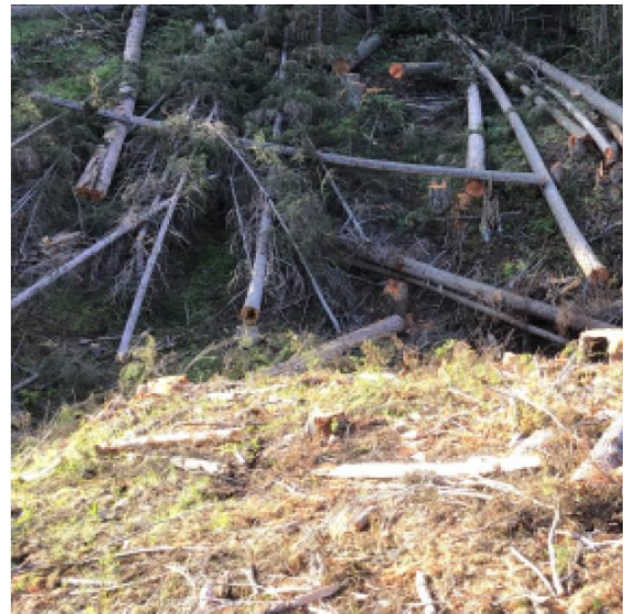
Timber removal using dozer and winch at Kingsvale Transmission Line. Timber will be removed and placed along the right-of-way to be processed and bucked for transport.
