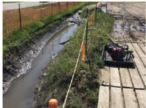
Generator positioned in secondary containment as a spill prevention measure.
