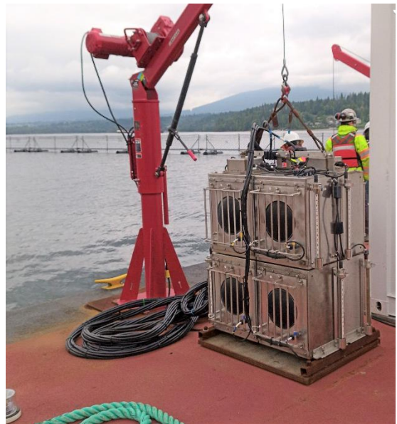
Fish deterrent system at WMT.
