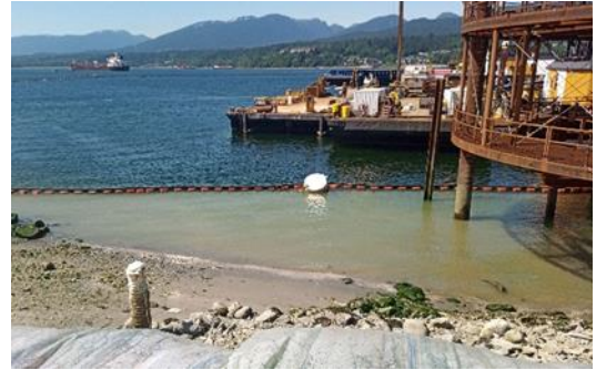
New turbidity curtain at the Westridge Marine Terminal foreshore.
