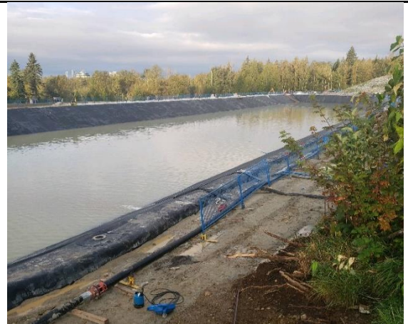
Intermediate Stormwater Retention Pond (ISWRP) at the Burnaby Terminal.
