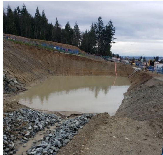
Stormwater collected into the Tank 97 holding area that will flow into retention pond.
