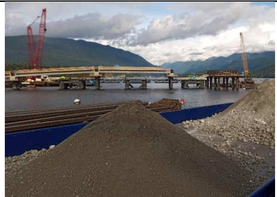
Grout spoils material on barge ready for transport to Trans Mountain approved off-site disposal site.
