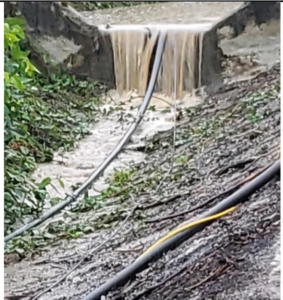
Existing constructed drainage canal at Burnaby Terminal facilitating management of erosion and sediment control on-site.
