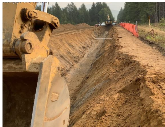
Excavation of pipeline trench off access road (Shoofly 23) near Norfolk Road, with topsoil piled on the side of the right-of-way.
