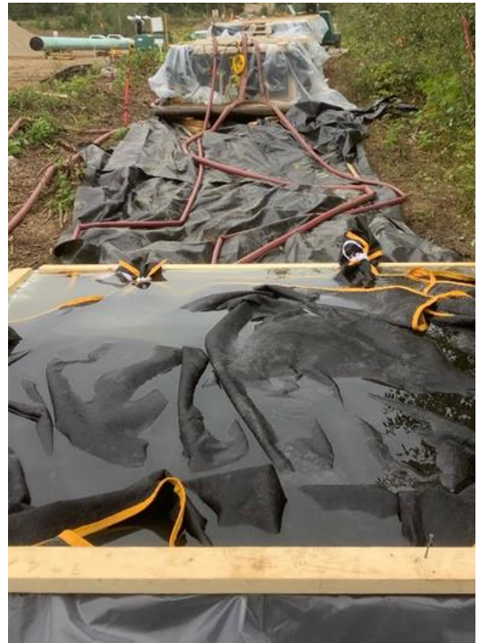
Pump-off structures used to filter water removed from excavations during pipe installation.
