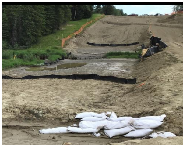
Erosion and sediment control measures including sandbags, silt fencing and snow fence near a creek.
