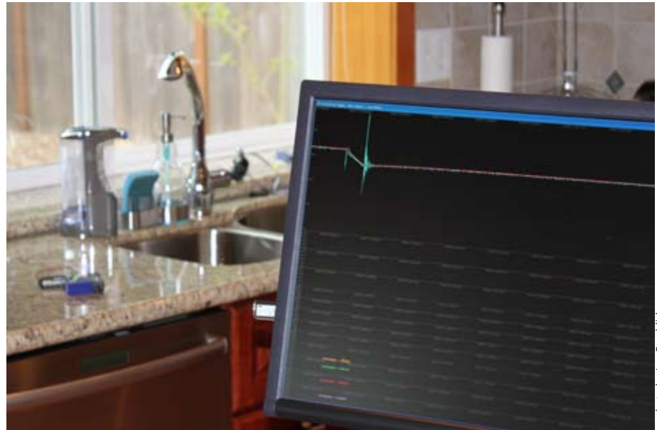
The monitor displays a HydroSense pressure wave created by using the kitchen faucet (background). Each water fixture in the home generates unique pressure waves, which travel throughout the home plumbing system, thus enabling the single-point sensing HydroSense approach.
